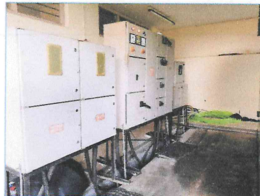
AC DISTRIBUTION BOX
