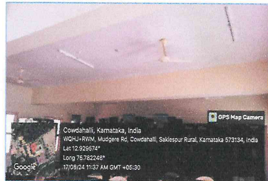
USE OF LED LIGHTS IN LIBRARY
